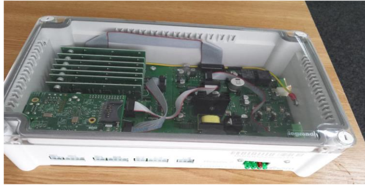
Figure 41 - Public Lighting Measurement and Control Module (MMC-SIP) used by the public lighting system in Bucharest
